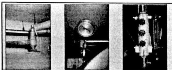
The above pictures show a Safety Relief Valve, a Steam Gauge and a Water Column in that order.
